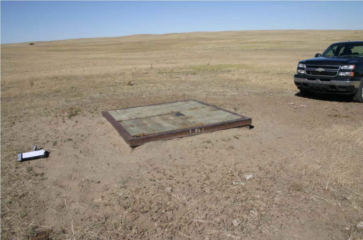
Figure 4. A 2000 well head installed in the NWA. Photo demonstrates the bare ground existing 6 years following development. Photo also demonstrates erosion found at surrounding the caisson, as the caisson was originally placed at ground level.
