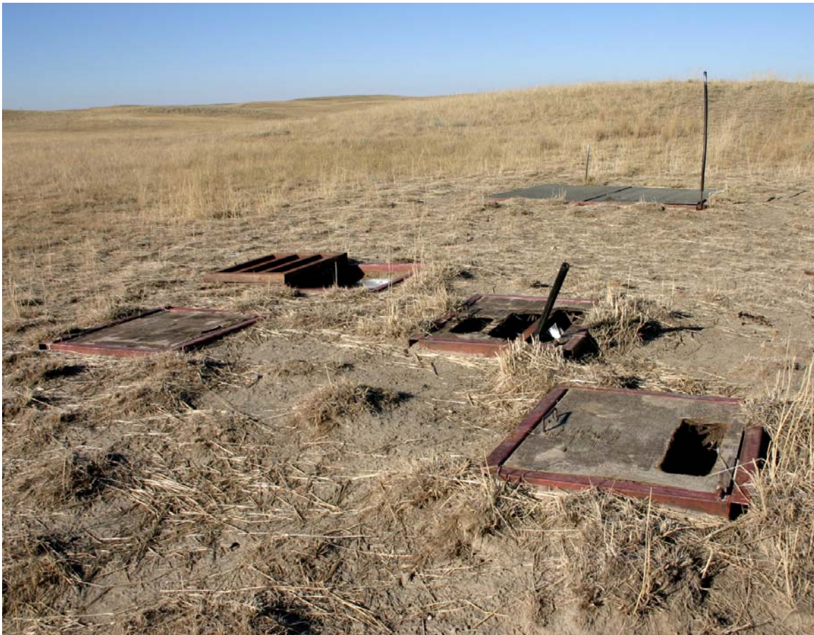
Figure 10. Photo demonstrates increased impacts of below ground gas infrastructure within the NWA. The rear of the photo is the below ground well head, where as in the fore ground are four shut-off valves for the pipelines. Note the poor state of the ply-wood cover, which can be a cause of wildlife injury as the mammals hoofs fall through the gaps while running past. Note as well that one of the shut-off caisson cover grates was left open, thereby creating a health and safety concern for all that access the NWA,
