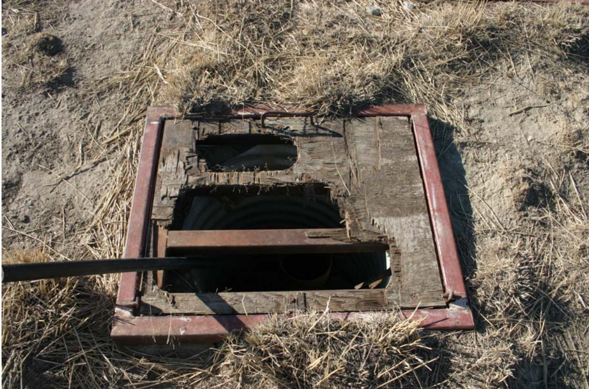
Figure 11. NWA 2006 photo of cover for a pipeline shut-off (isolation) valve demonstrating the poor ply-wood cover. This is an up close image of a portion of Figure 10.
