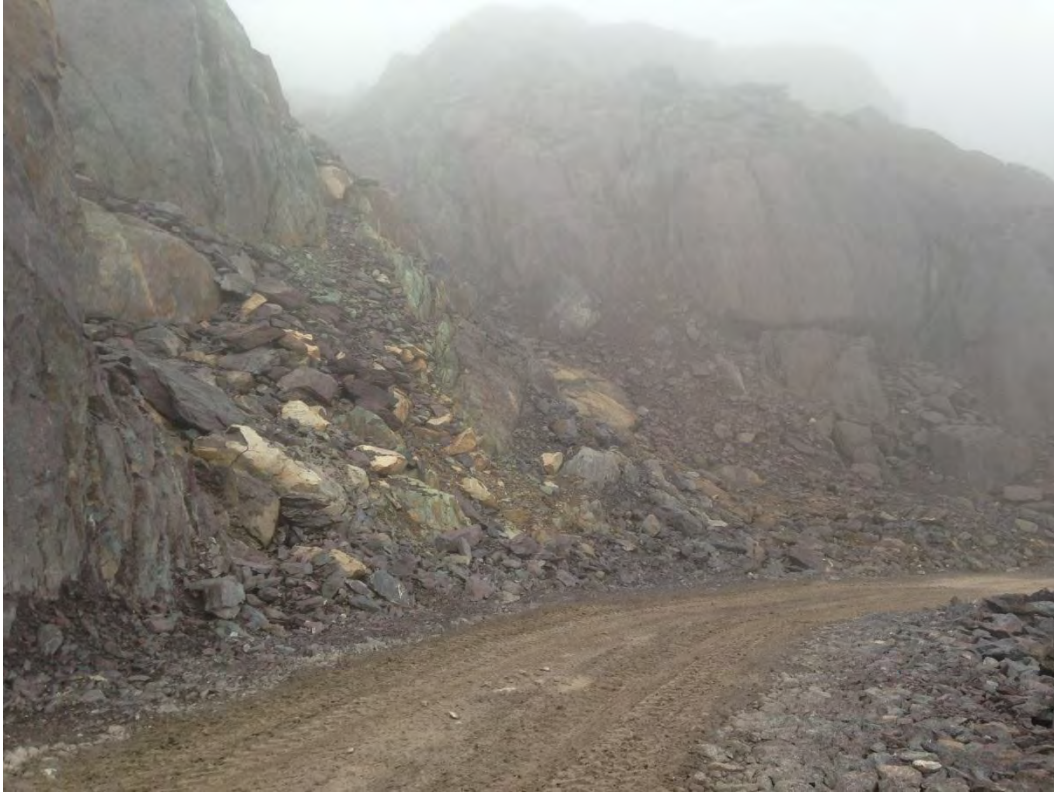
Photograph 3-2. Area of rockfall hazard along access road at approximately KP 72. Photograph by BGC, looking west.
